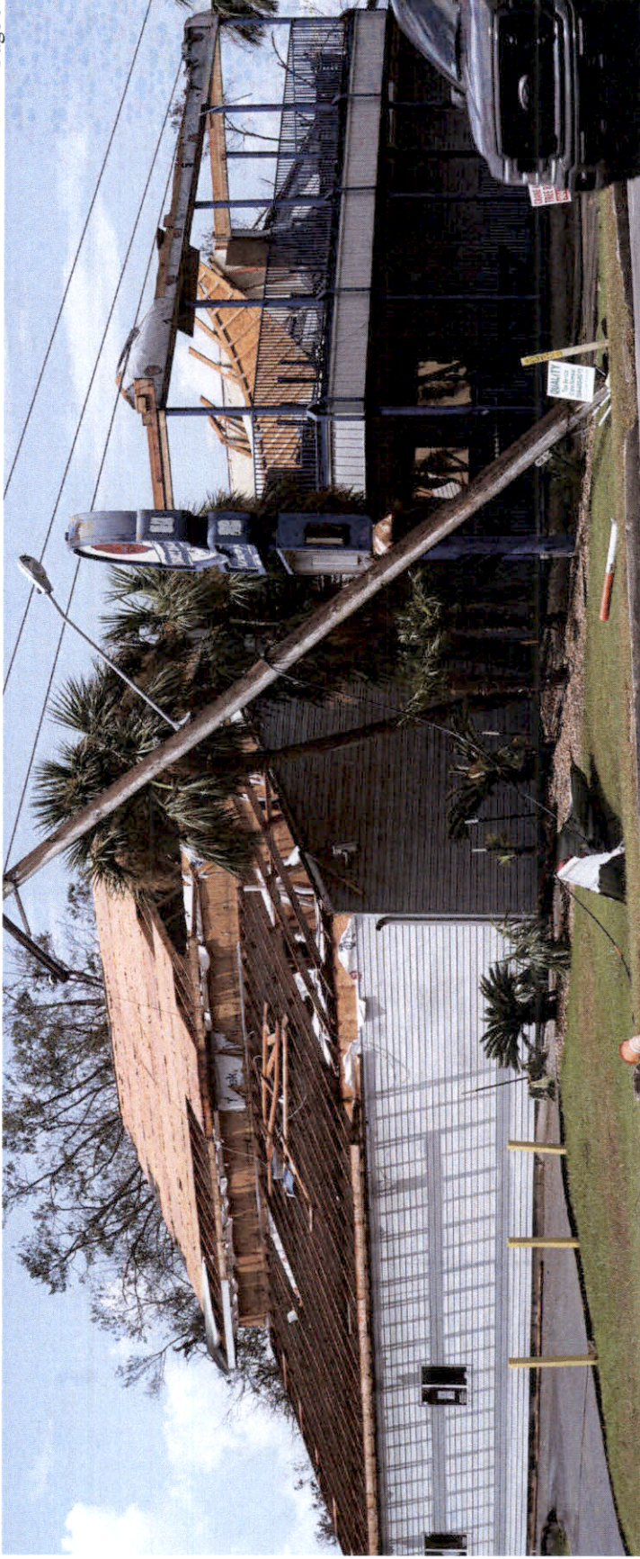
Leaning distribution pole next to building with significant roof damage
