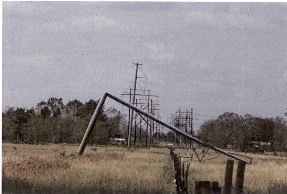
Figure 4-4. Steel Structure Failed above the Groundline
