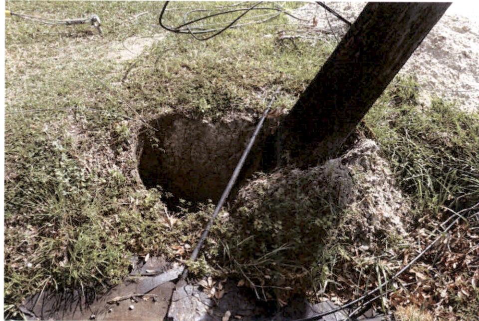
Figure 4-10. Displaced Soil at Base of Pole
