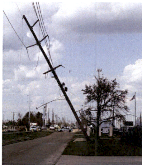
Figure 4-9. Wood Pole Leaning Due to Soil Displacement
