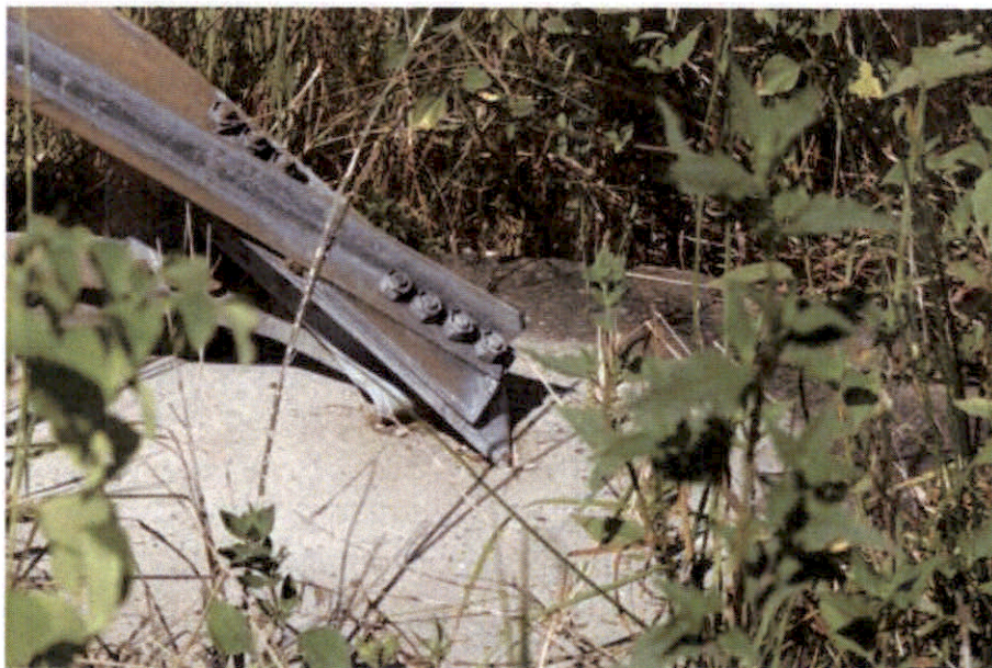
Figure 4-3. Close-up of Stub Angles Bent Over at Foundation on Structures
