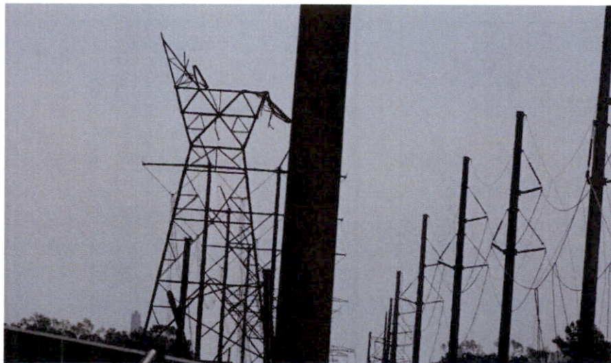
Figure 4-7. Steel Structure Damaged at the Top of the Structure
