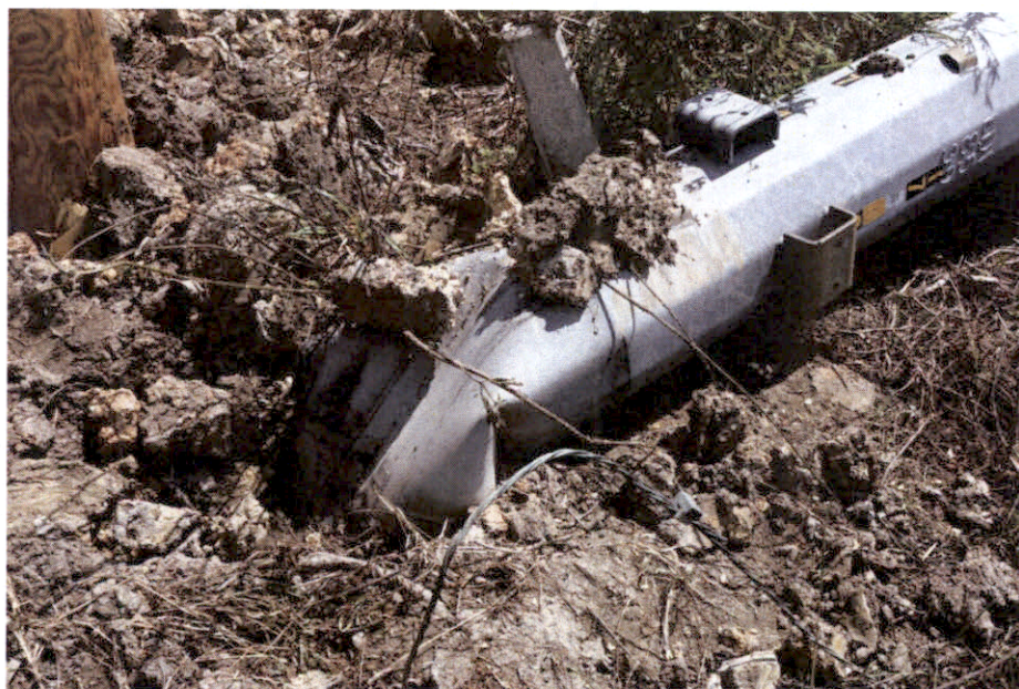
Figure 4-5. Steel Pole Bent at the Groundline
