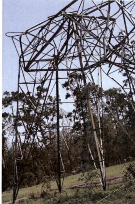
Figure 4-6. Steel Structure Failed at the Waist
