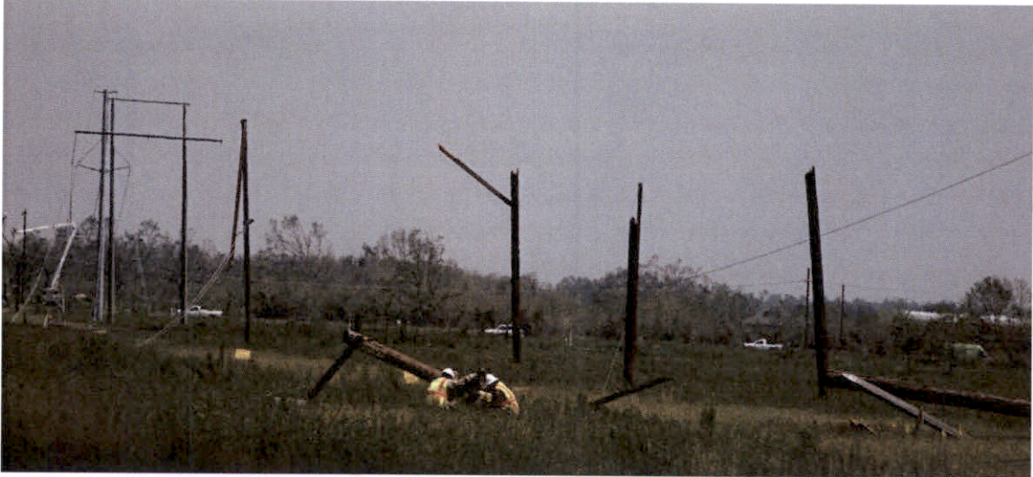
Figure 4-8. Wood Poles Destroyed above the Groundline
