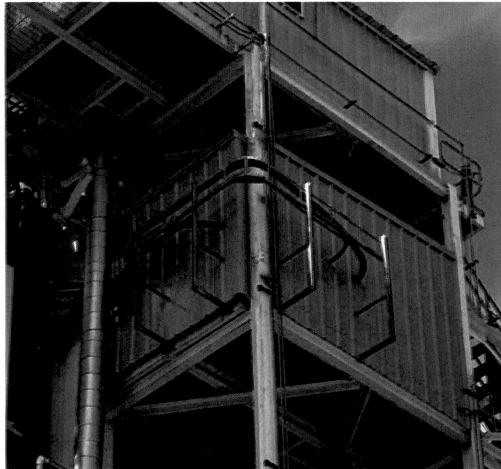
Figures 5 and 6: Drum Level Transmitter Enclosure
